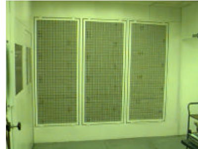
Figure 8.- Air Replacement Unit
